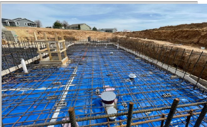
Pump area of equipment building - foam, vapor barrier, rebar and floor drains installed
